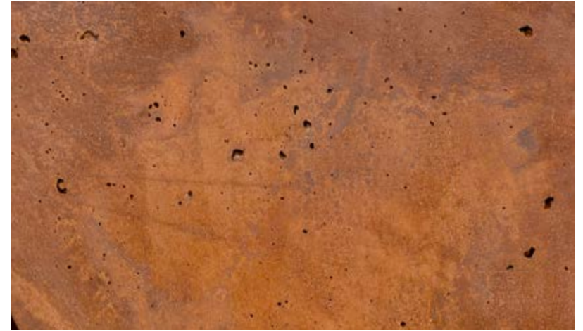
FERRO CONCRETE aspect rouillé
